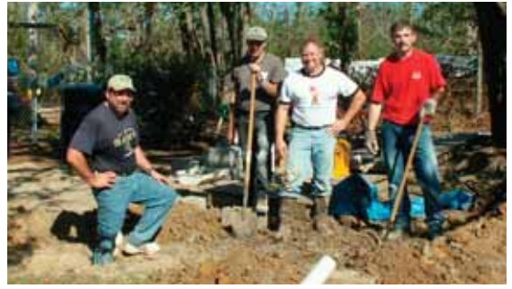
Randy Schmidt, Dave Potts, Jed Scheuermann and Mark Lindquist fixing a broken sewer line.
